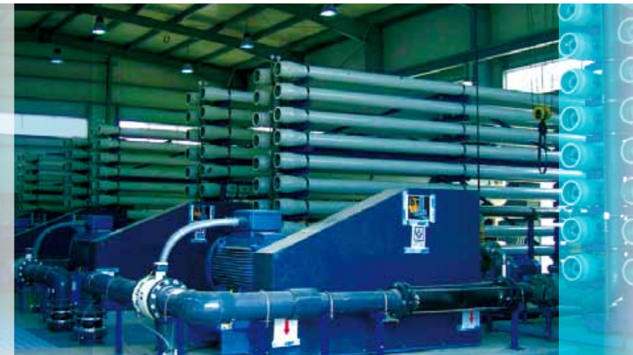
High energy efficiency seawater RO system
