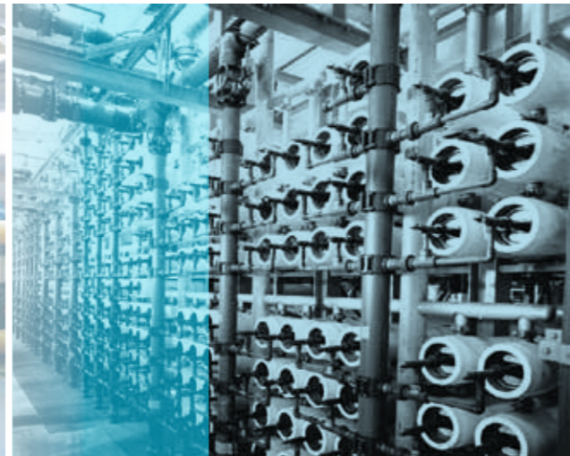
High recovery seawater RO system
