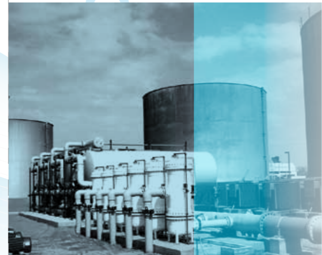
25,000 m3/day seawater RO pre-treatment system
